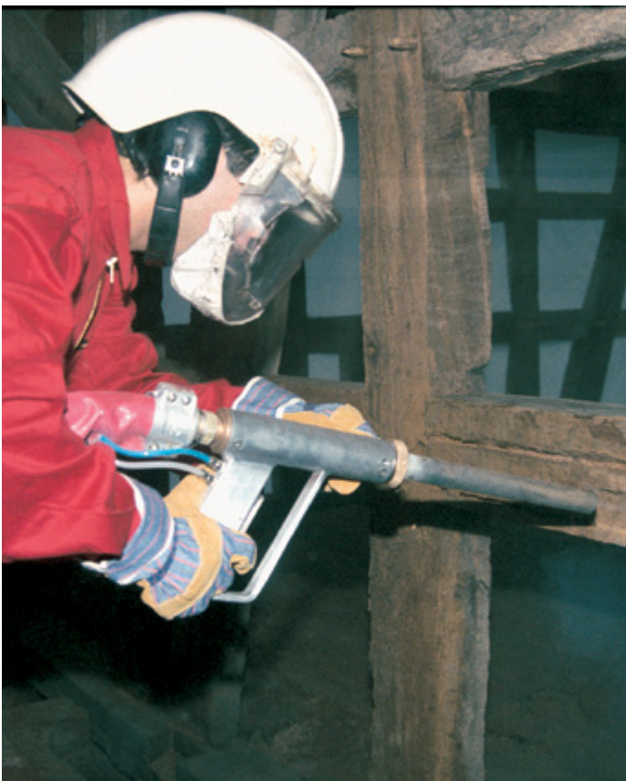
When dry ice blasting (e.g. when renovating an old half-timbered house, as shown here), always wear protective clothing.
